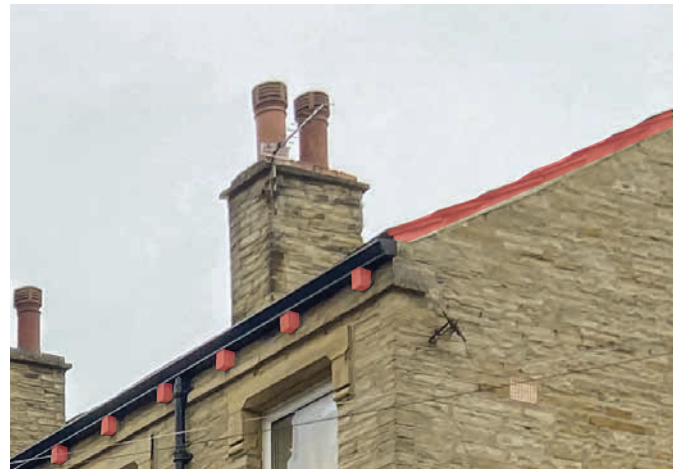
A consistent roof design with wet verge and stone dentils supporting the gutter
