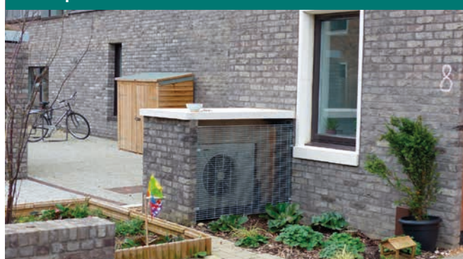
Air source heat pump for a residential building - Marmalade Lane, Cambridge.
