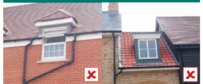
The poor placement of dormer windows results in rainwater downpipes dominating the composition of the elevation and awkward and ugly detailing
